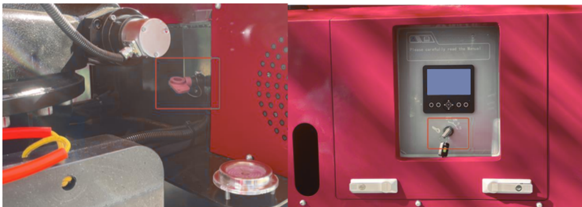
Figure 2. Main power switch
